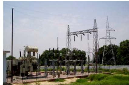
Chilwaria cogeneration: power export to the grid
