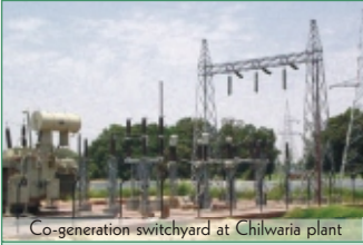
Co-generation switchyard at Chilwaria plant
