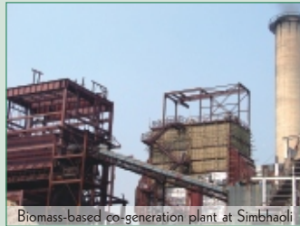
Biomass-based co-generation plant at Simbhaoli
