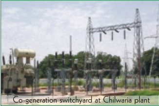
Co-generation switchyard at Chilwaria plant
