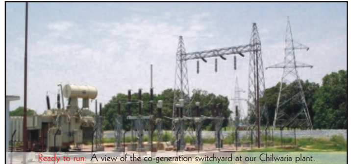
Ready to run: A view of the co-generation switchyard at our Chilwaria plant.
